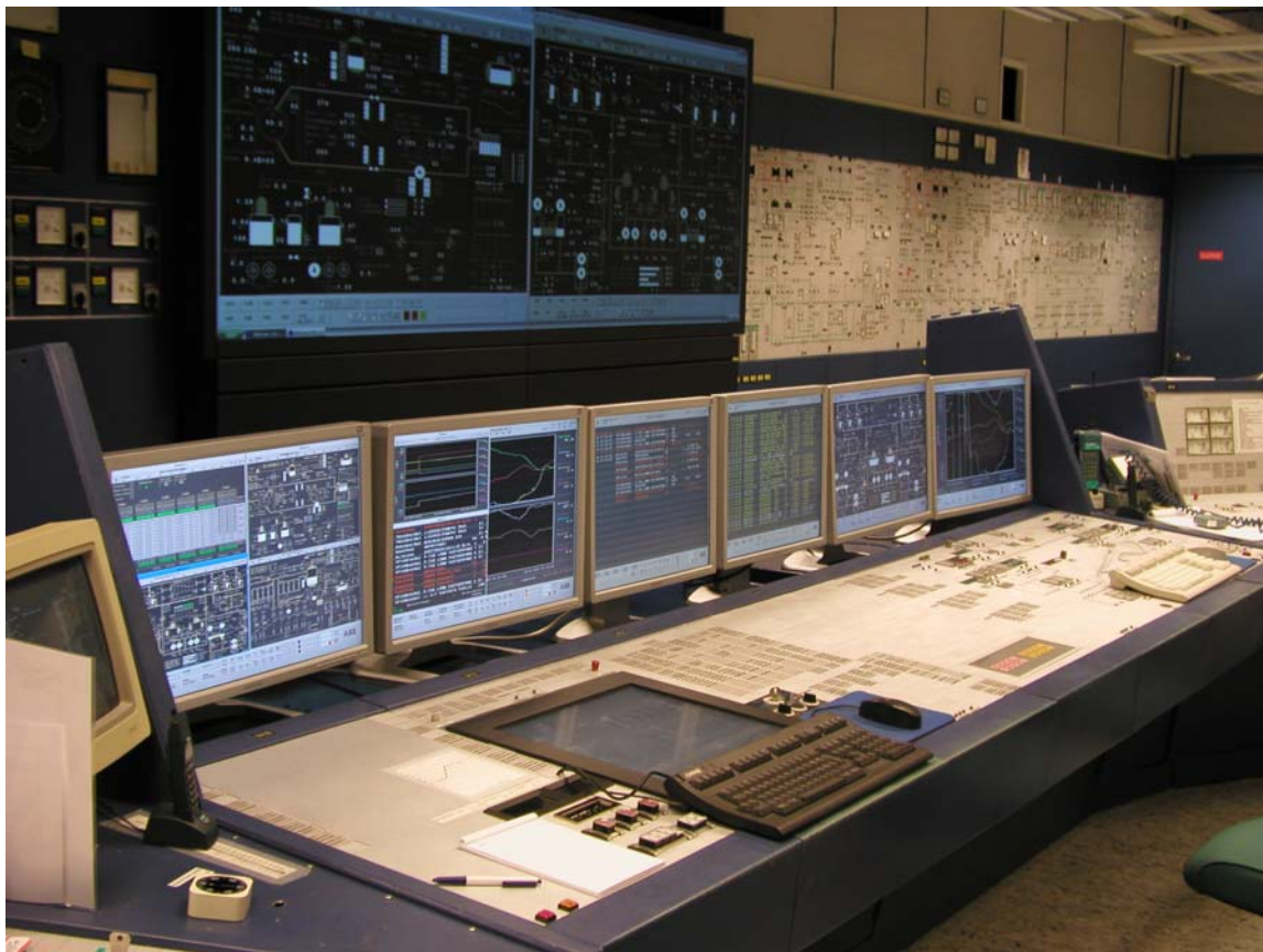
Picture 2. LOTS in January 2007 after upgrade to LARA stage 1. In the front the QDS display is installed in reactor operator's desk and in the back two large screen display elements are presented.
